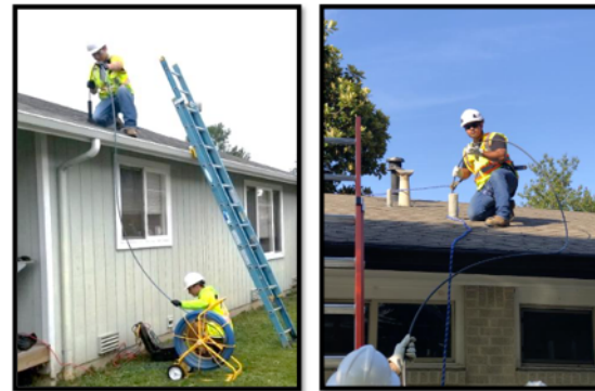
Figure 20: Roof vent inspection with manual push camera. Fall protection must be used according to safety regulations.
